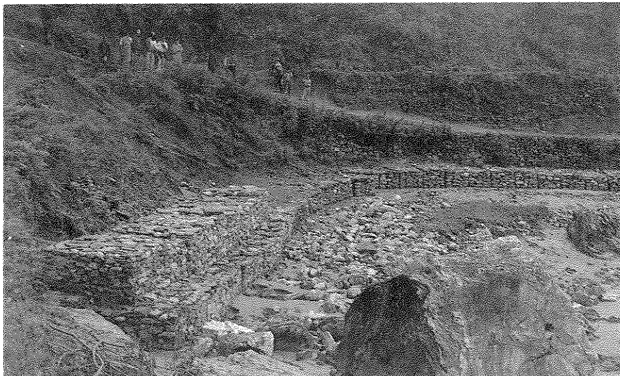
Photograph 8D Gabion Revetment to Prevent Toe Cutting of Hill Slope by River Flow
