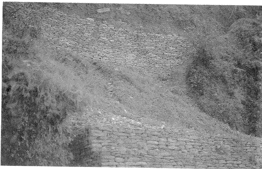
Photograph 8B Gabion and Dry-Stone Retaining Walls to Stabilise and Reduce the Risk of Land Mass Failure
