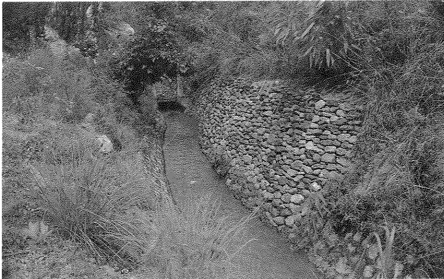
Photograph 8C Dry-Stone Revetment Wall to Stabilise the Cut Slope and Prevent Minor Landslides
