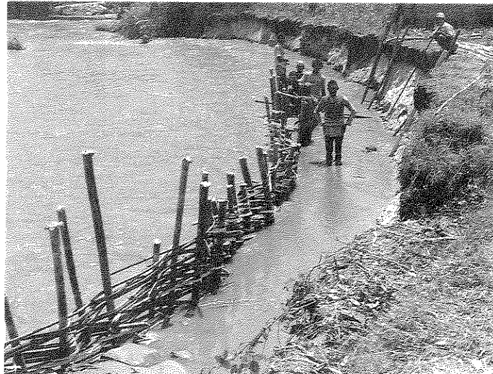
Photograph 6A Sandbag Revetment Behind Rows of Bamboo Piles Protecting River Bank from Further Erosion
